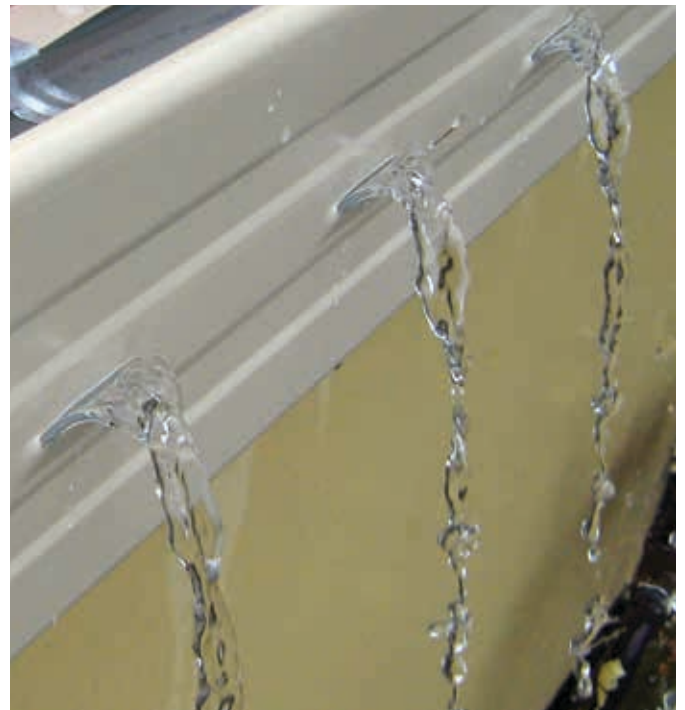
Typical overflow from slotted gutter.
